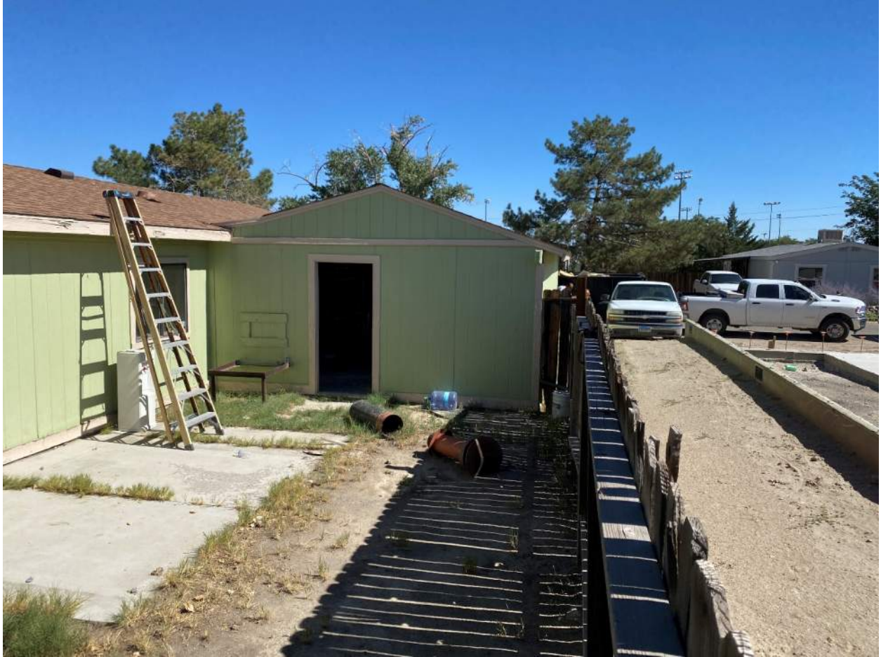
Looking easterly along south property line at garage proposed for zero lot line setback, with recently completed foundation on southerly adjacent 395 Parkland Avenue
